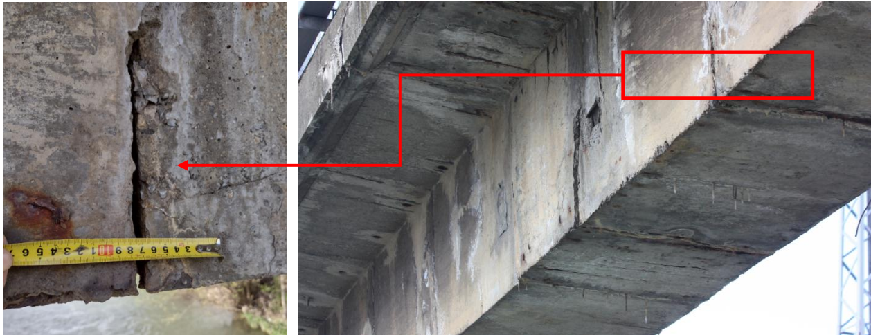
Fig. 2. Opening of the joints between the segments in the middle of the second span
