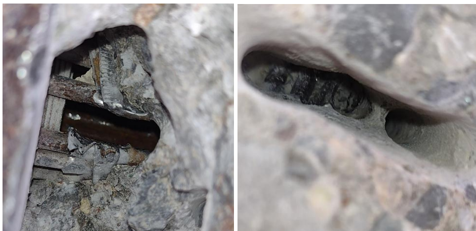
Fig. 6. Non-grouted prestressing tendons in the bottom slab of the precast concrete; left – anchorage point, right – approx. 0.5 m behind the anchor
