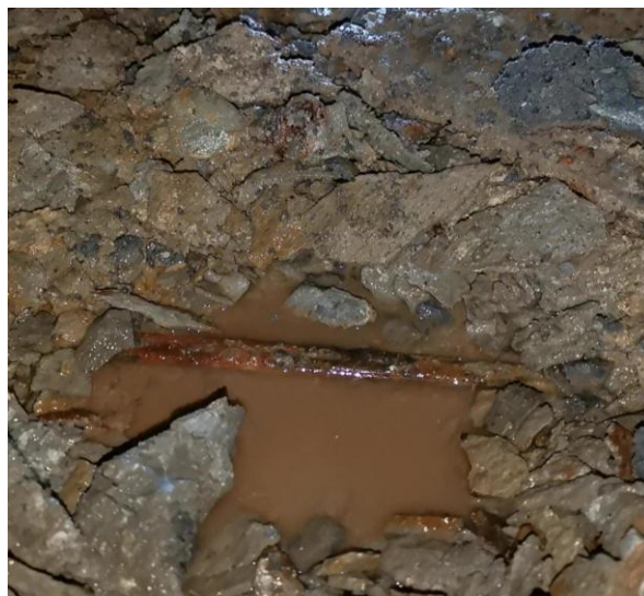
Fig. 3. Corroded prestressing reinforcement
