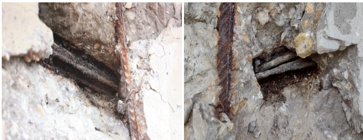
Fig. 4. Non-grouted cable ducts with corroding prestressing reinforcement
