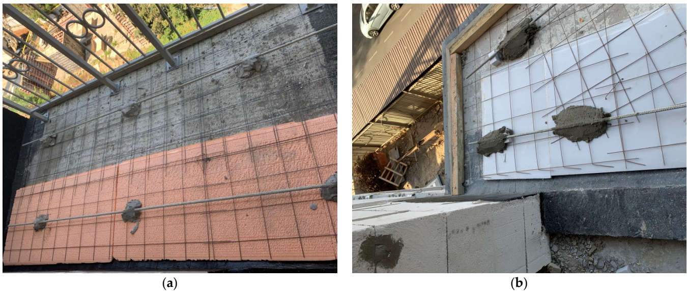
Figure 9. Installation of insulation of balcony floor slabs in accordance with research results at facilities in the city of Odesa: (a) loggia, (b) balcony.
