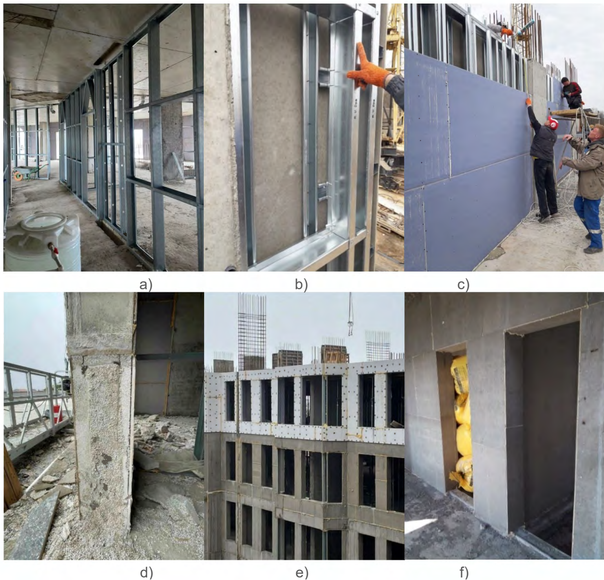
Figure 11. Process of erecting the developed solution of the enclosing frame structure using expanded polystyrene concrete in a fixed formwork: a) erecting the frame from LSTWS; b) assembly nodes of the frame from LSTWS; c) sheathing the frame with cement chipboards; d) concreted wall; e) external view of the finished structure from the outside of the building; f) external view of the finished structure inside the building
