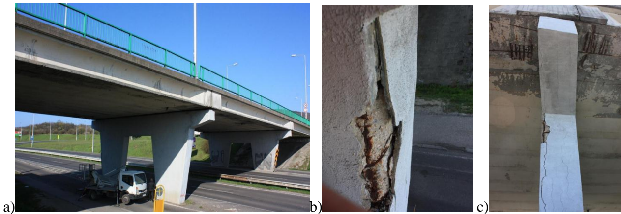
Fig. 3. View of the bridge (a); condition and failures of the substructure (b, c)
