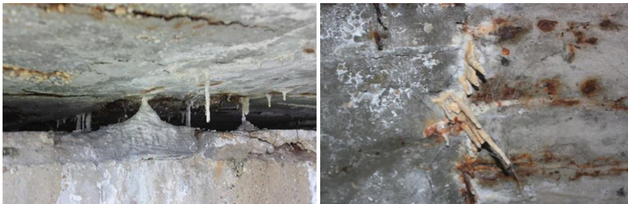
Fig. 5. Intensive leakage of the structure
