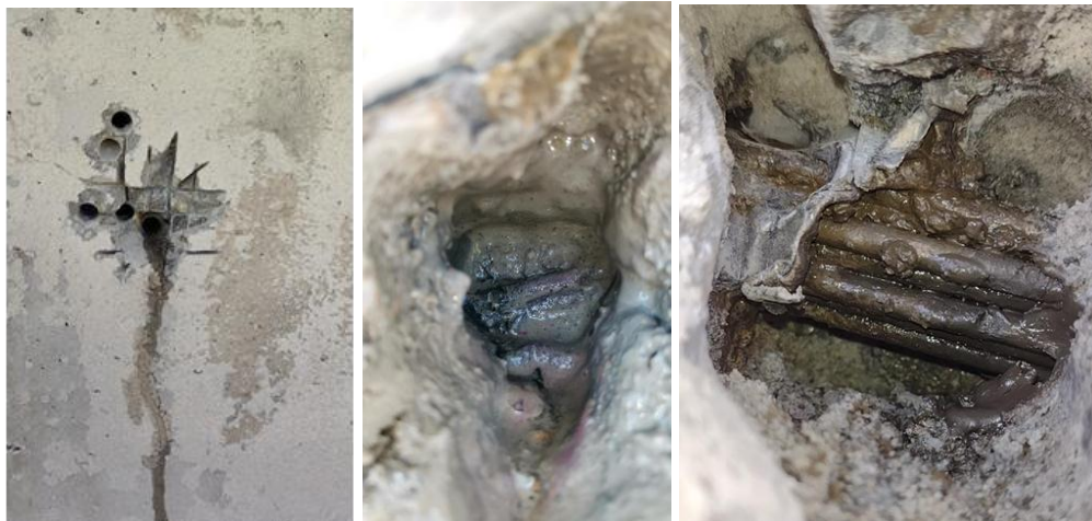
Fig. 6. State of prestressing reinforcement in tendon ducts from which water leaked after drilling
